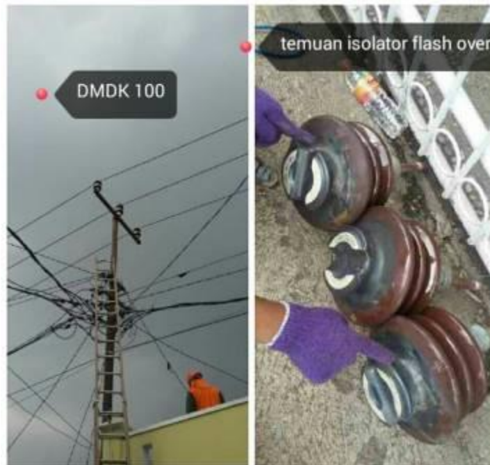
Gambar 4. Gangguan Akibat Isolator Flash Over
