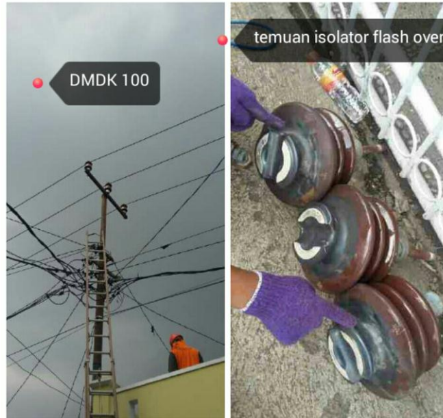
Gambar 4. Gangguan akibat flash over
